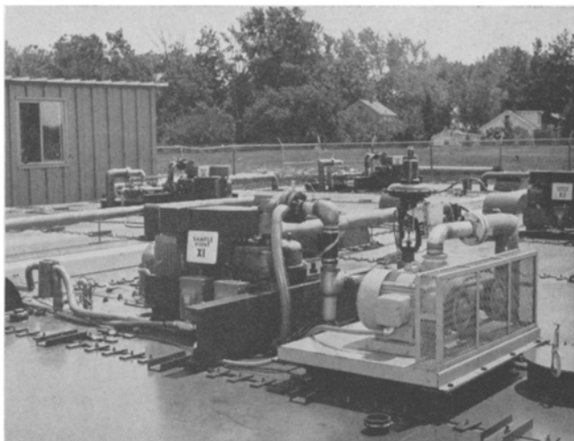
FIG. 6. View of stage no. 1 oxygenation system aerator, blower and turbine drive.
